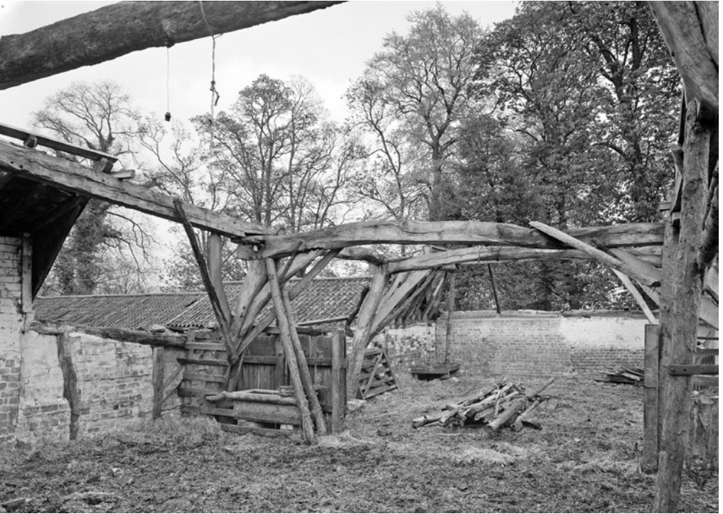
Figure 8.1. Building at Ketsby, Lincolnshire, UK. A view looking eastwards to the north side. Photographer unknown, 1966. Historic England Archive. Reproduced with permission.
