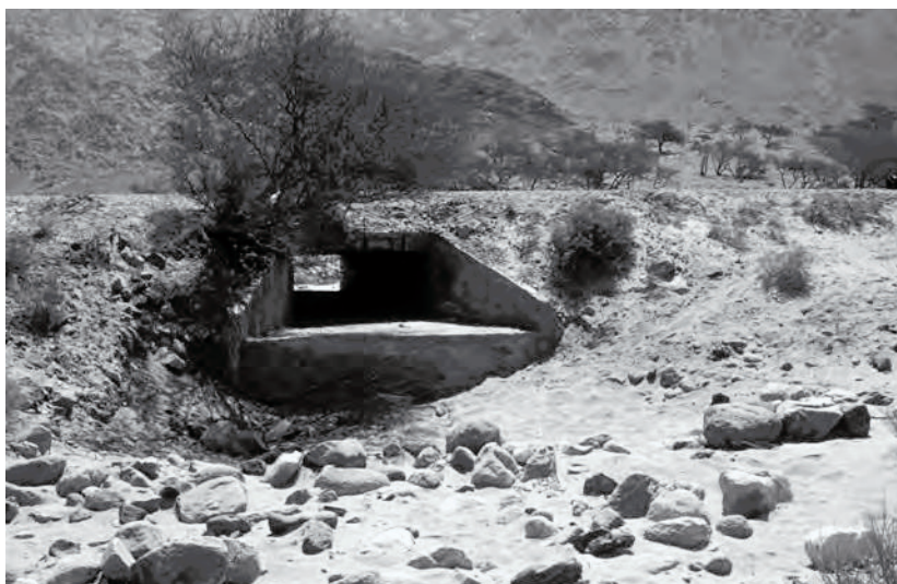
Figure 15.15: A culvert installed underneath the Dead Sea Highway channels a large volume of seasonal runoff directly towards Structure A001: view from the west (photo: R.J. Cook).
